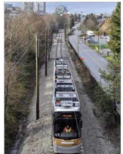
PNR RailWorks constructs the Olympic Line, a demonstration street car put into operation during the 2010 Winter Olympics.
