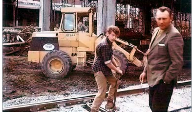
George Braun, Sr., (foreground) and Henry Braun (on loader) work on Project 2000 for CP Rail, which later becomes the site of Canada Place and the Vancouver Convention Center.
